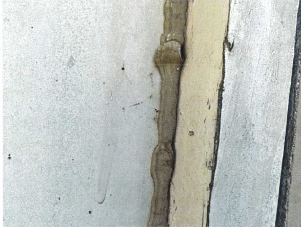
FAI-204-100223-013, 014, 015 None Detected, White Caulk
